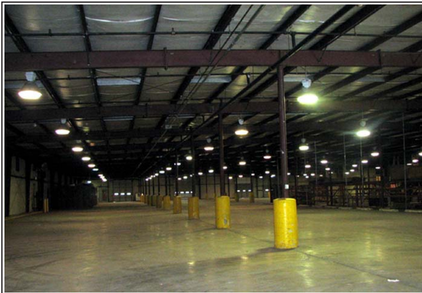
Located in Pike County, the interior view of the Hobbs Warehouse is shown above.
