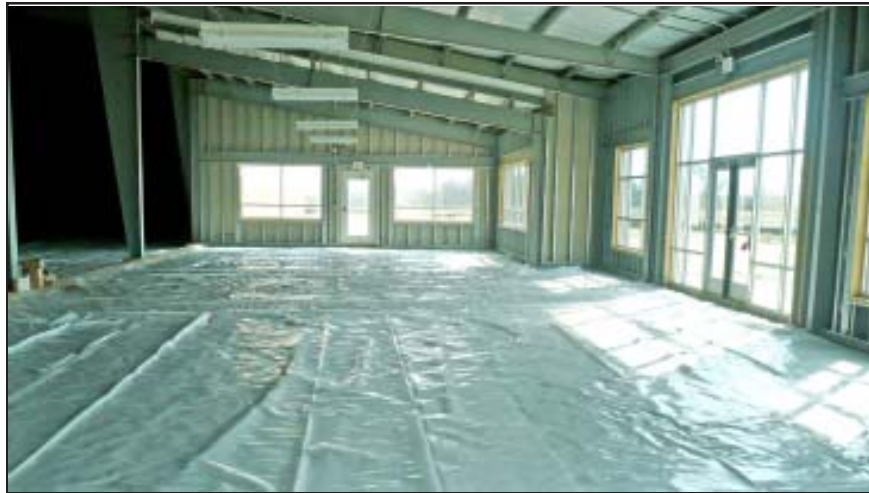
The interior view of the Russell County Speculative building is pictured above.
